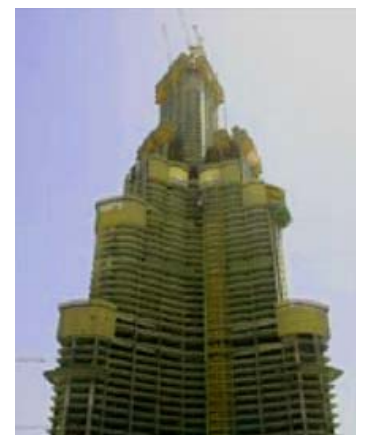
The Burj Dubai will contain the world's highest elevator installation.
